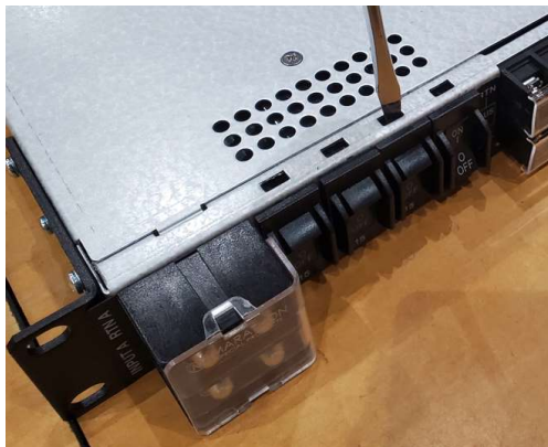
Figure 2: Breaker Replacement Slots
